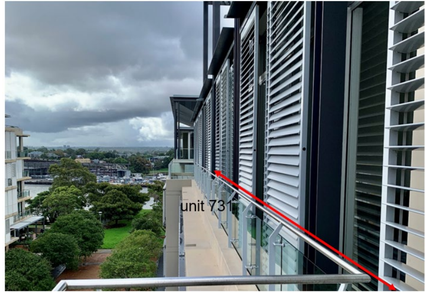
west elevation of unit 731 - viewed from western end of the private terrace
